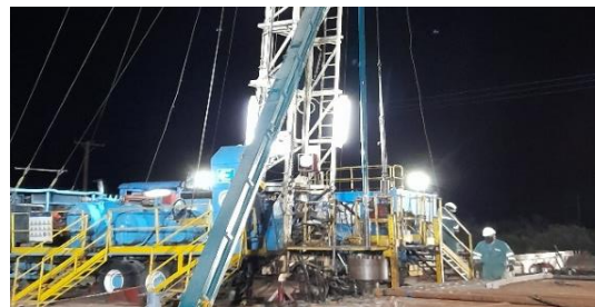
Lifting a beam for an ESP install.
