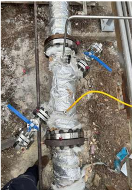
Original ultrasonic flowmeter
