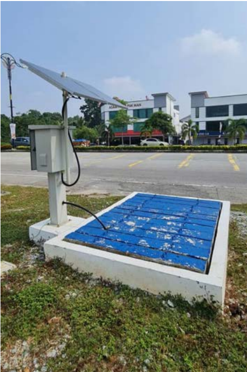
Fig. 2: Solar panel powering the AT600 battery in the cabinet which connects to the IP68 C-RS 401 transducers underground
