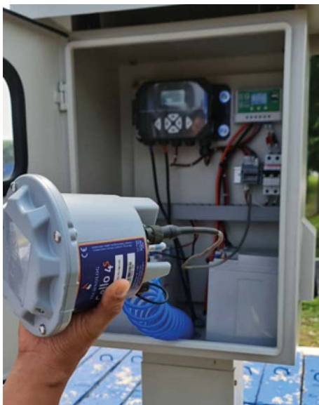
Fig. 1: Cabinet with AT600 electronics, data logger, battery and 4G communication module
