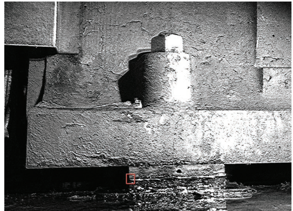
Example of soft foot detected on a reciprocating compressor
