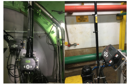
Fig. 3: AT600 and AT20 installation on two of the lubricating lines
