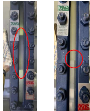
Condensate carry over volume visibly high while using incumbent chemical (left) and no carryover while using DMW1414 (right)
