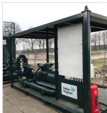
Centrifugal pump skid.
