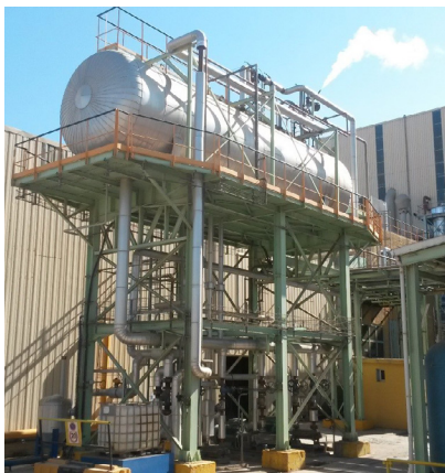
Condensate recovery vessel and downstream circuit of the condensates at the GRD-LaBelle plant
