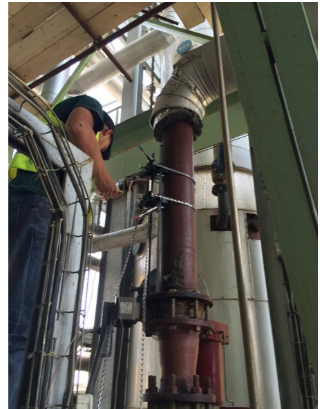
Flow measurements at condensate inlet and outlet
