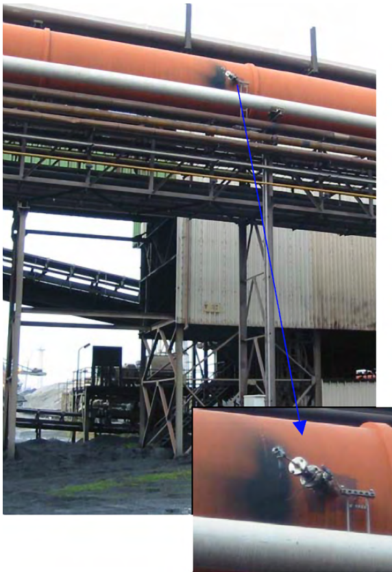
Figure 2. Customer installation site
