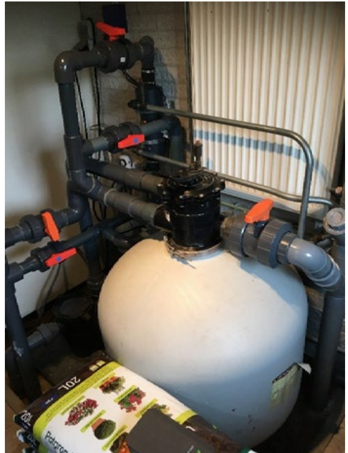
The complete filter installation
