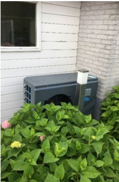
The 20kW heat exchanger
