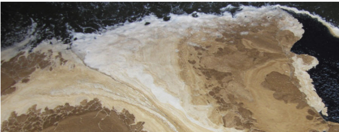
Hydrocarbon leak in cell one of north cooling tower basin.
