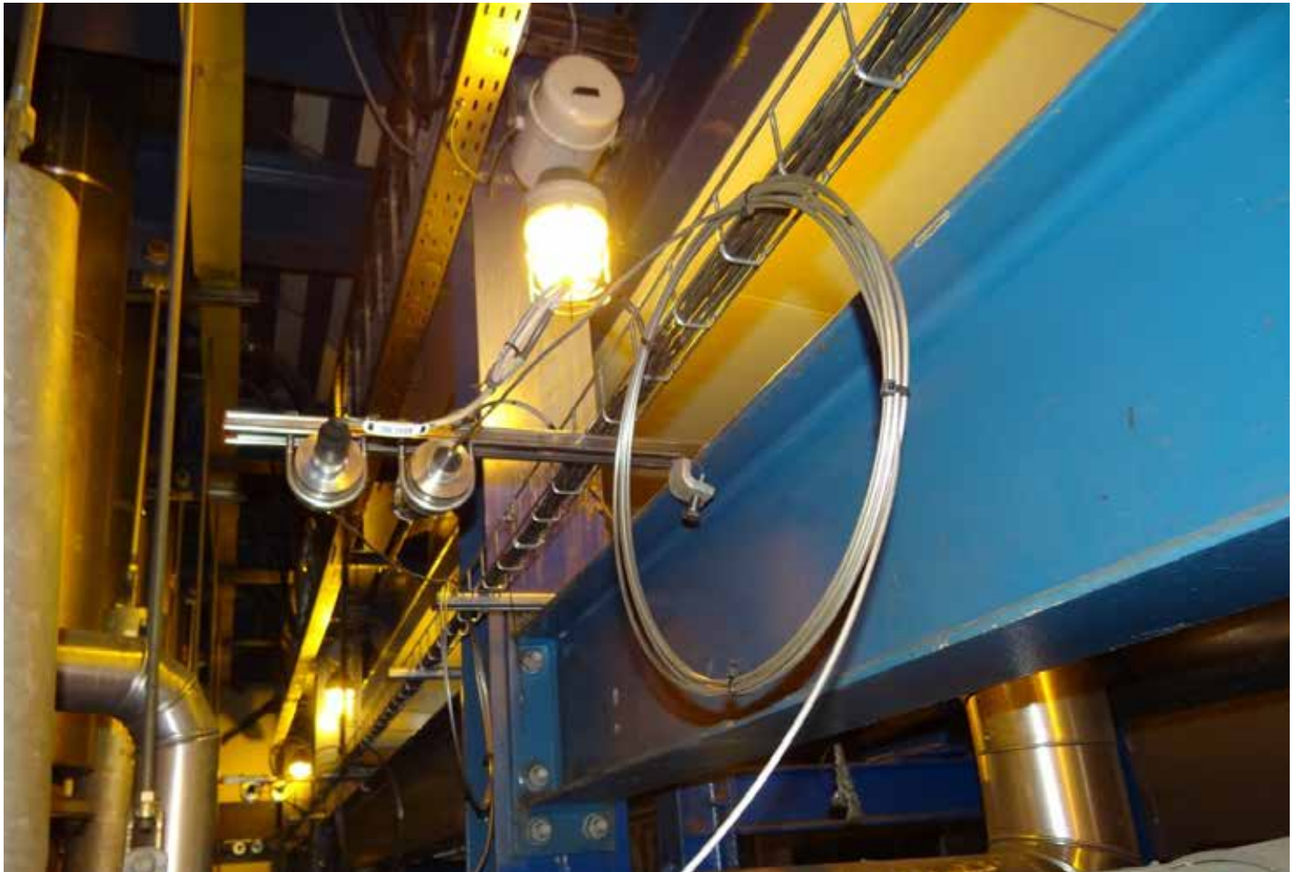
Figure 4 – FTD 325 cool ends with excess MI cable in a loop
