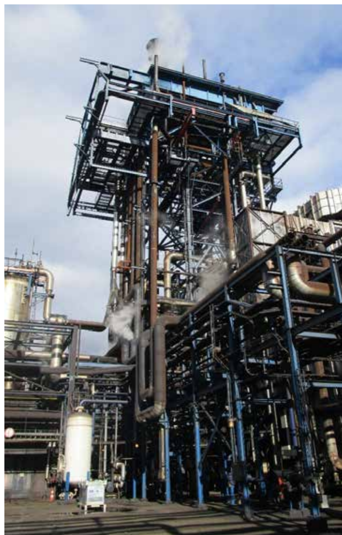
Figure 1 - Yara Tertre Steam Methane Reformer
