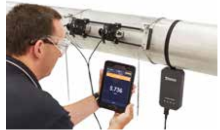
IMAGE 2: Portable flow meter in use
