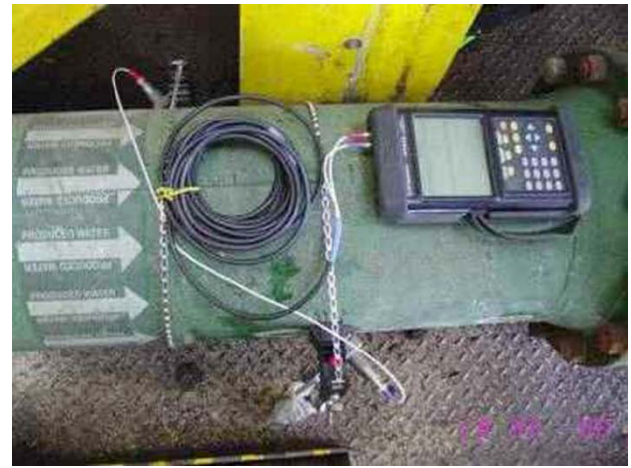
PT878 in use on 12-inch Produced Water line, with insertion-turbine 3D downstream
