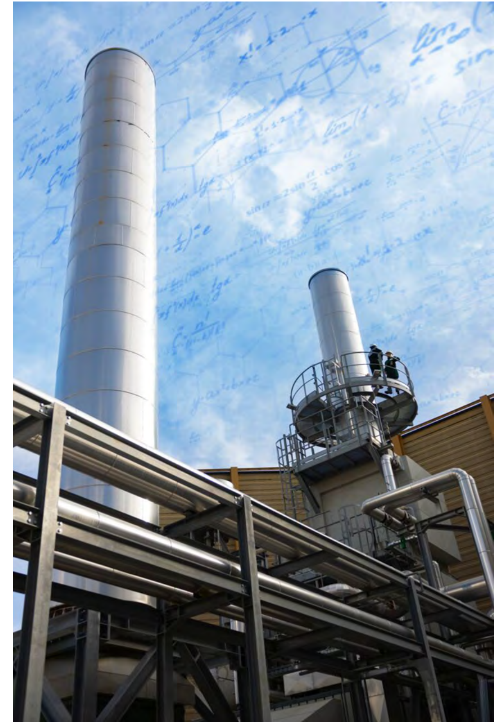
Co-generation area, Florence, Italy
