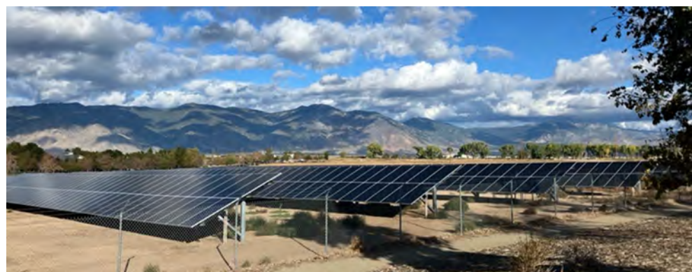
Baker Hughes facility Minden, NV U.S.
