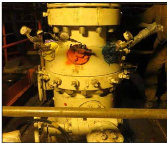
Figure 18—XMas Tree Termination
