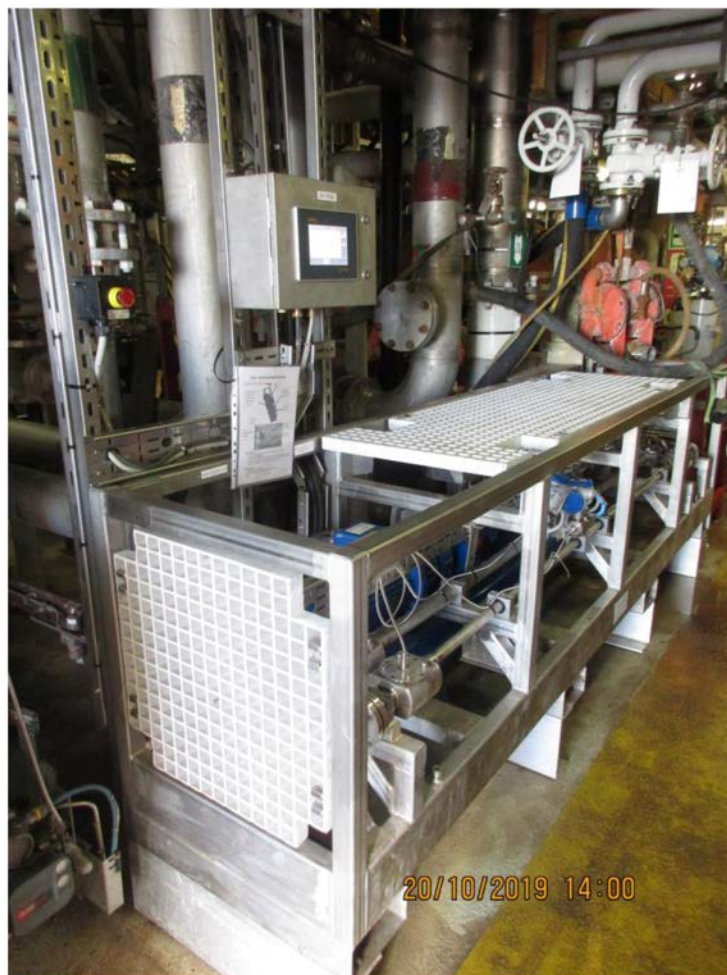
Figure 2—AFM unit installed on an offshore platform in Norwegian sector
